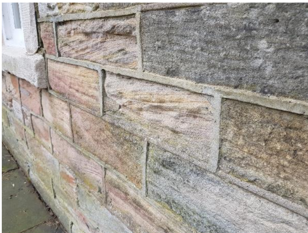
Figure 84. Ribbon pointing with cement is resulting in damage to the softer stonework
