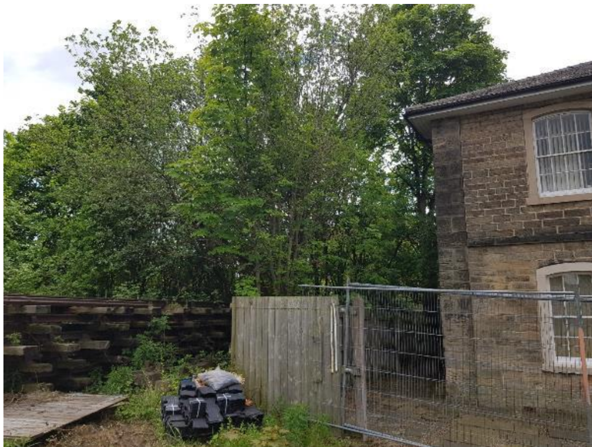
Figure 85. Self-seeded sycamores are too close to the building and could cause root damage and restrict ventilation
