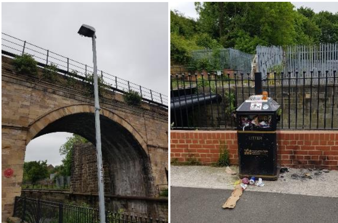
Figure 71. Left: The current lighting is an unwanted intrusion in photographs of the bridge. Also visible, vegetation growing along the parapets. Right: The bins need emptying more often.
