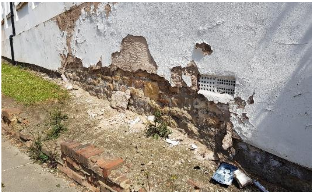
Figure 94. Failing render and paintwork on the carriage works leading to damaged stonework
