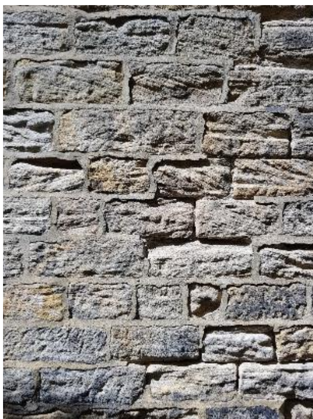
Figure 80. Cement has been used to repoint the building in the past. This has damaged the stonework on the Goods Shed. This photo is of the east elevation wall.
