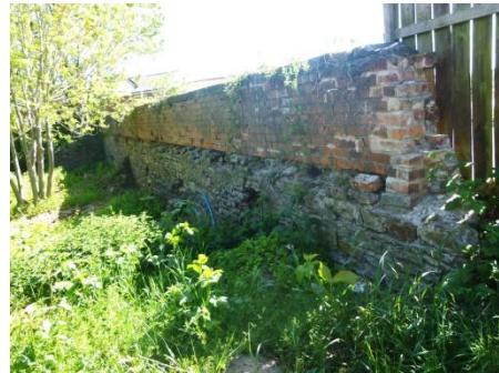
15 The coal drop wall needing repair
