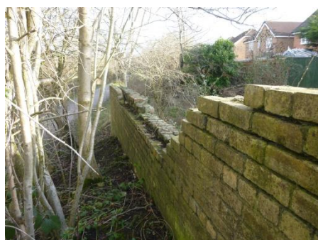
10 Old Station wall; damaged eastern end
