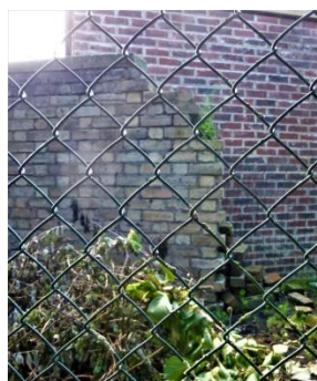
11 Old Station wall; damaged western end
